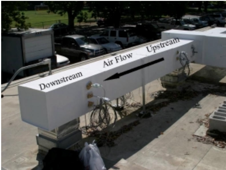
Figure 1: Configuration of sensors on either end of duct
