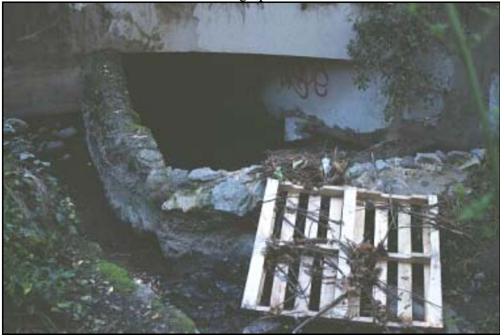
Looking downstream, on the left is the bypass channel, on the right is the box culvert
