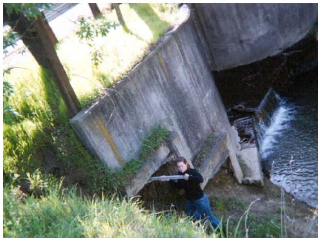
Figure 4. Erosion at downstream end of Alhambra Avenue bridge, right bank. 3/3/02.
