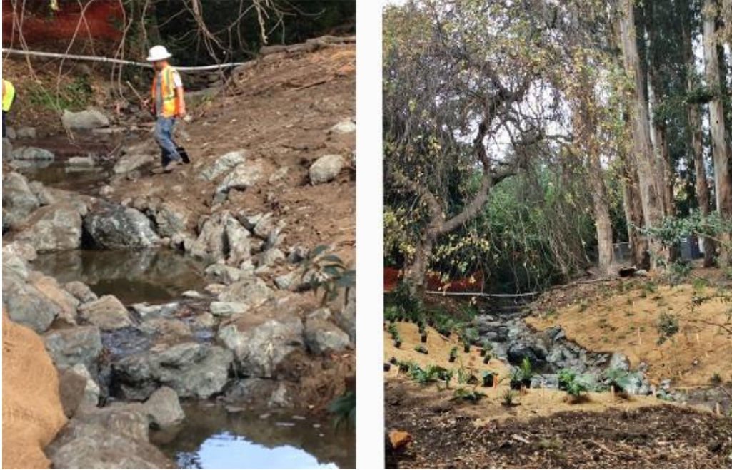
Figure 2. Left photo shows the construction of the step pools on the UC Berkeley campus in October 2014. Right photo shows the completed step pools in early November of 2014, with planned riparian vegetation waiting to be planted.
