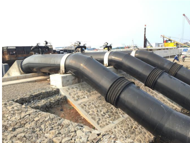
Figure 6*: Pluit pumps that pumps water out of Jakarta into the Java Sea.
