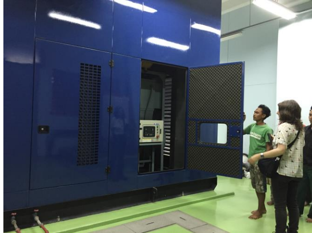
Figure 8: Generators for the pump, following the February 2015 flood incident, where the pumps failed because of electricity from the power grid was shut off.
