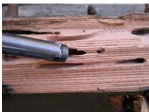
Photo: 27 - Drywood termite damage, Incisitermes , family Kalotermitidae Photo: Dr. Vernard R. Lewis
